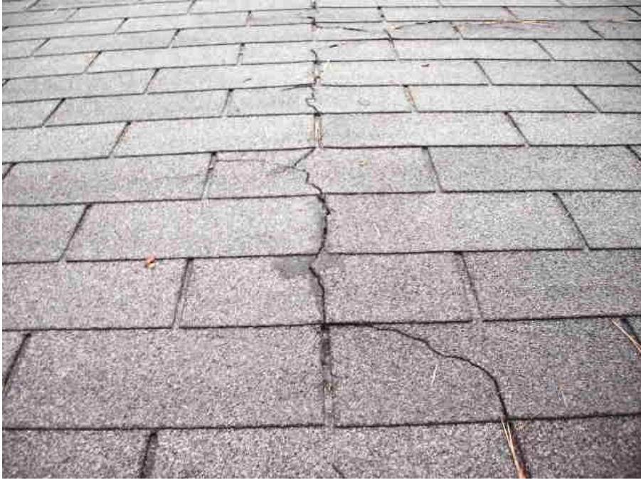
This close shows how the crack ran completely through the shingles
