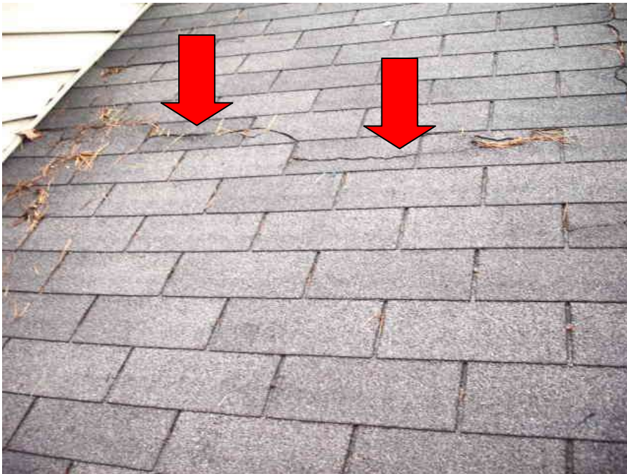
Some random horizontal cracks were also noted
