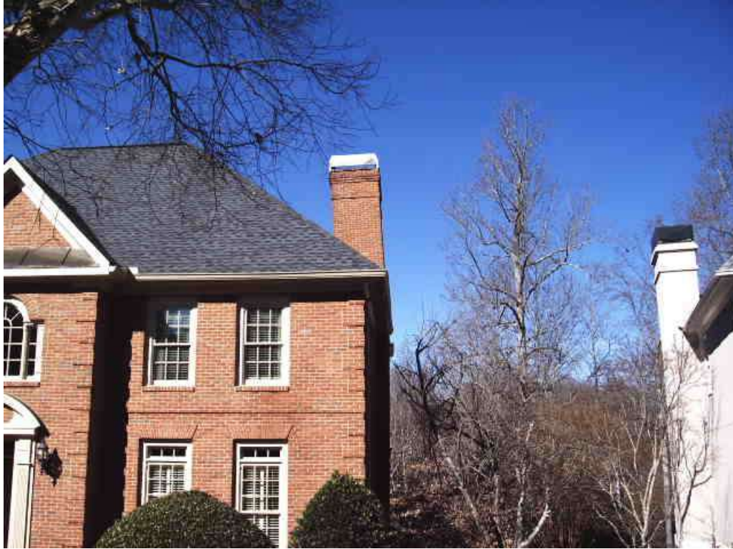
The chimney chase on this house is leaning in, towards the house.
