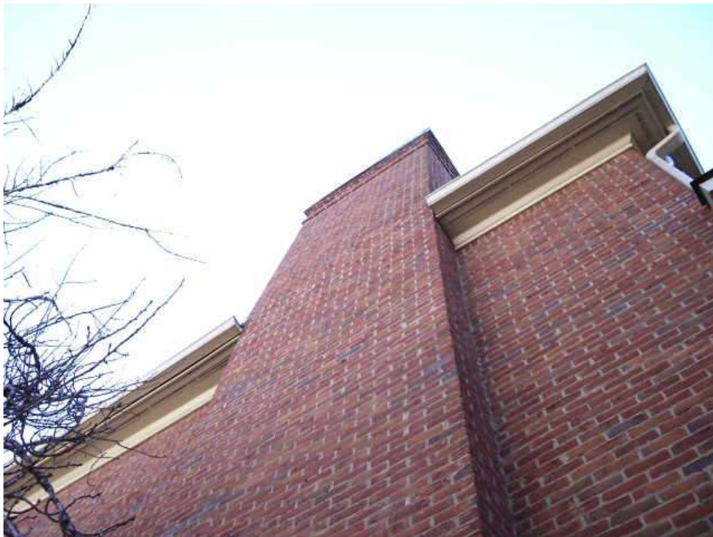
Looking up the chimney chase from the ground, one can see how it leans in
