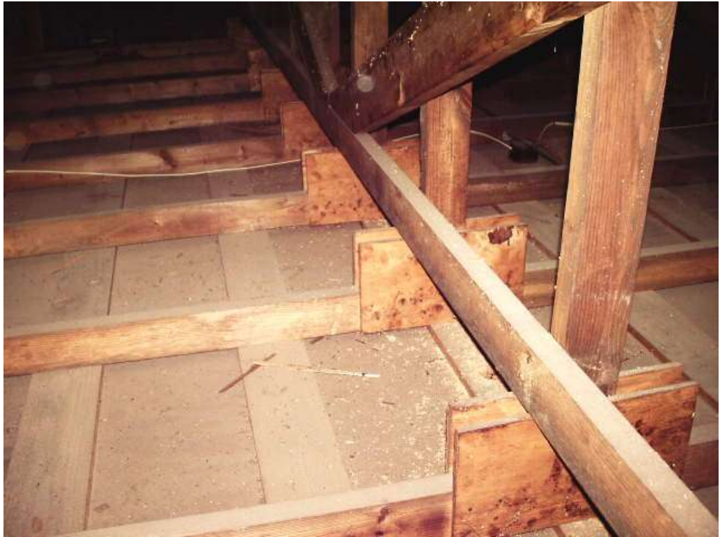
Gussets at the bottom of the vertical struts in the middle of the trusses.
