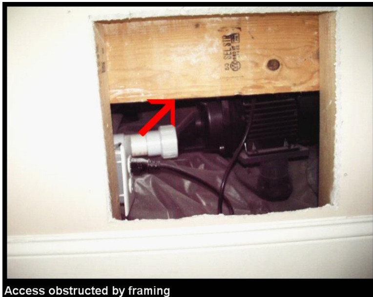
Access obstructed by framing
