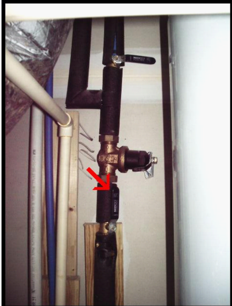
Main shut off
