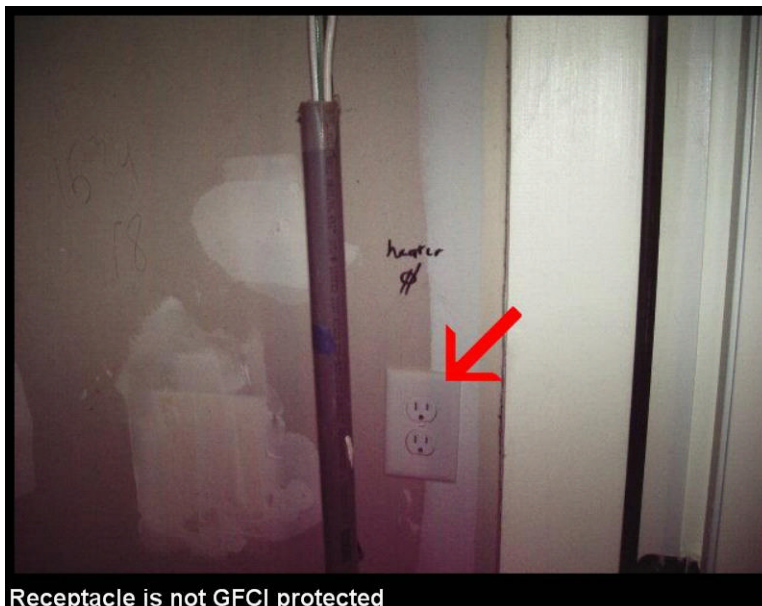
Receptacle is not GFCI protected
